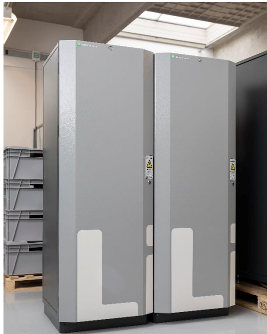
Figure 5. Two racks of battery modules.
