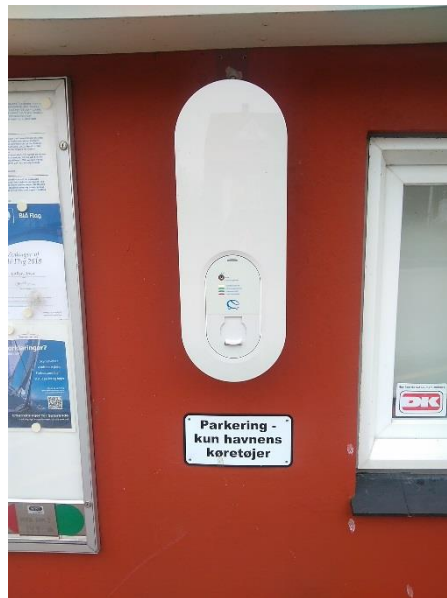
Figure 10. Charging point for the marina staff's electric car.
