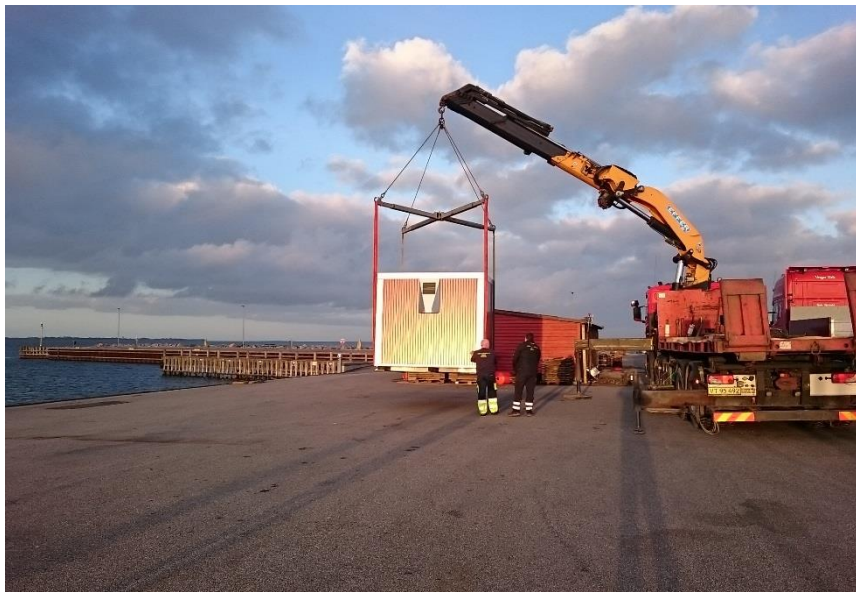
Figure 4. The cabin arrives on the marina. It is now inside the red Warehouse (background).
