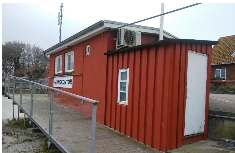
Figure 8. A new heat pump (below the roof edge) heats the harbour master's office.
