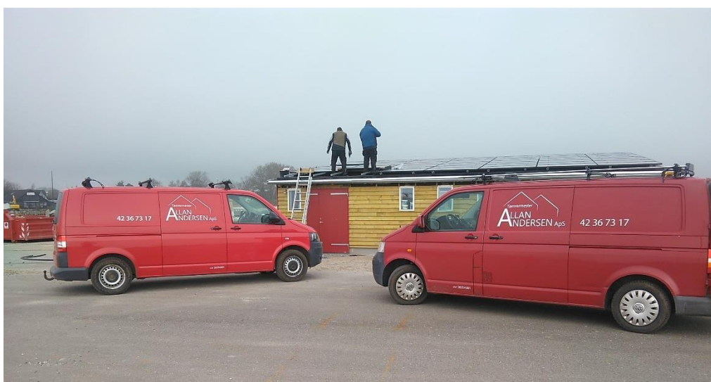
Figure 7. A local installer mounts PV panels on the Warehouse building, building 3 of the 'marina site'.
